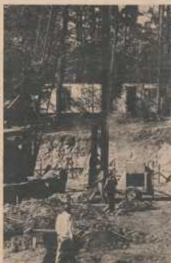
Expressway construction continues as ASDU and ECCOS negotiators with the State Highway Commission for environmental concessions.
